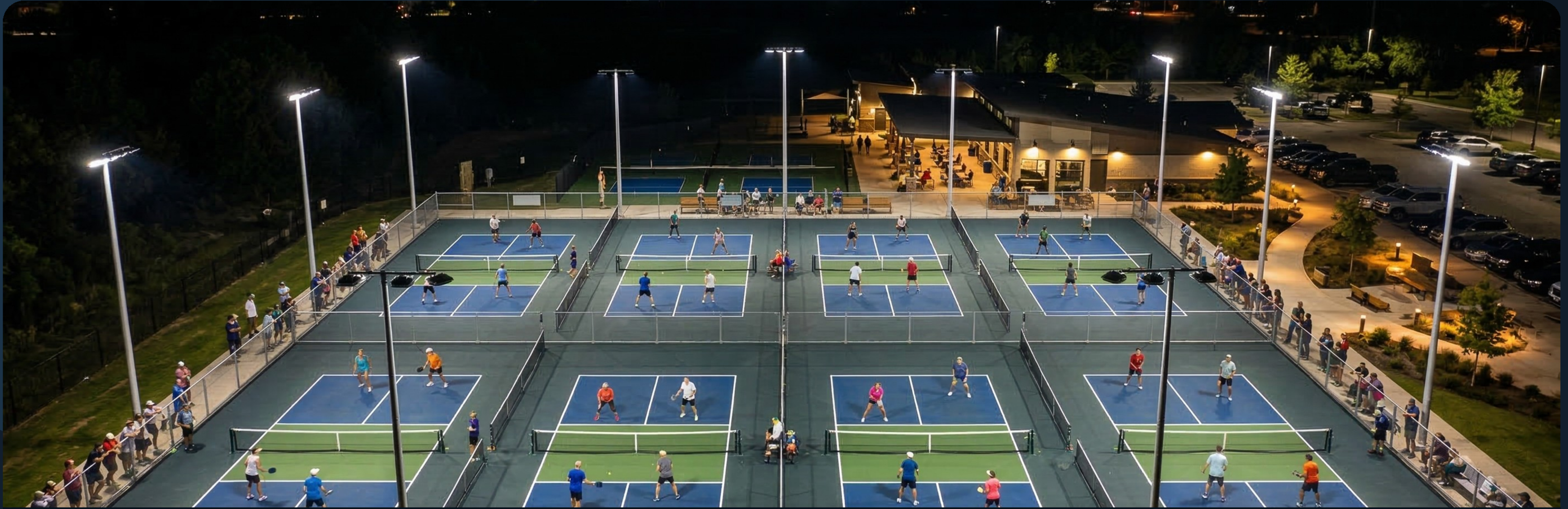
OUTDOOR FACILITY LIGHTING
