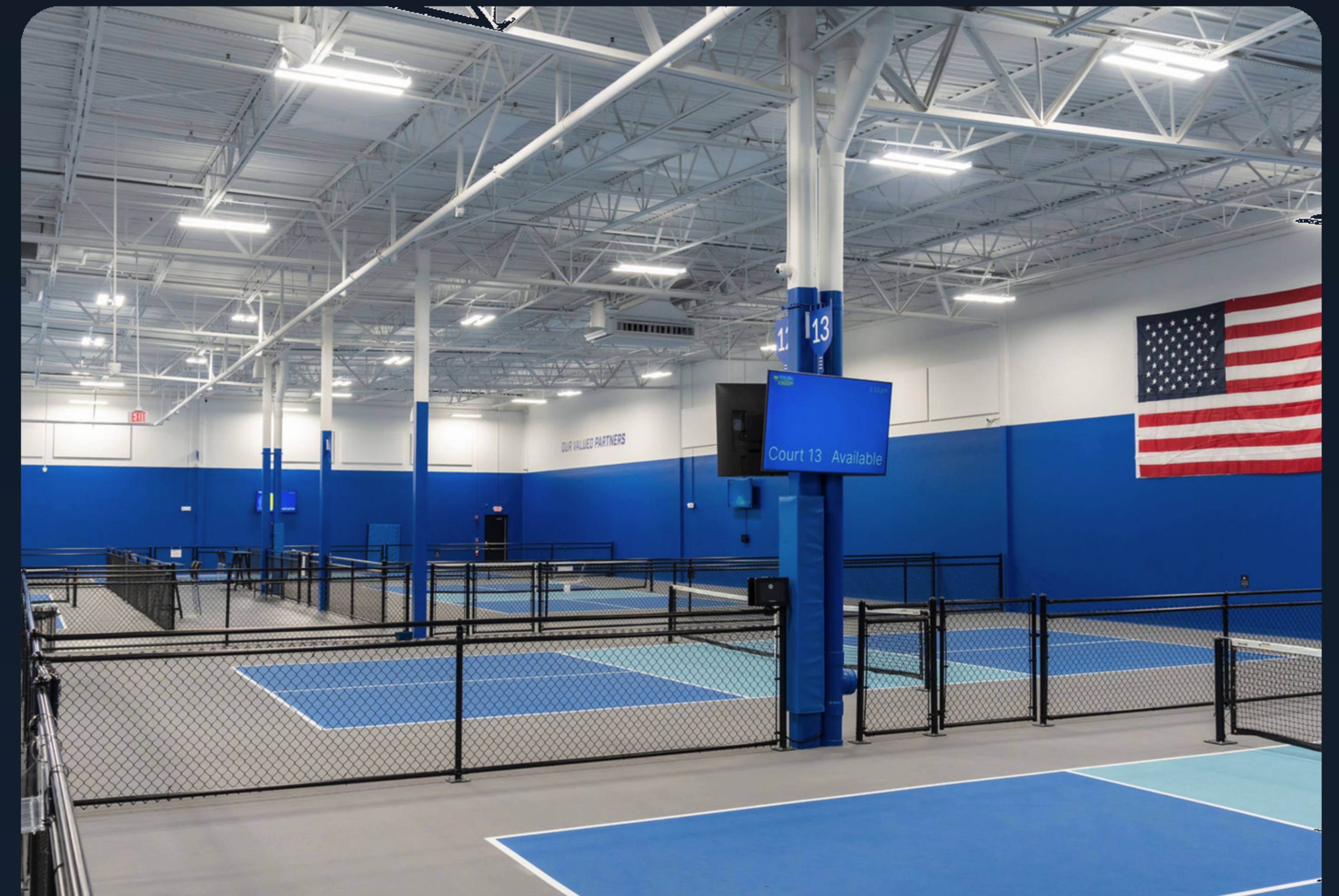
INDOOR FACILITY LIGHTING
